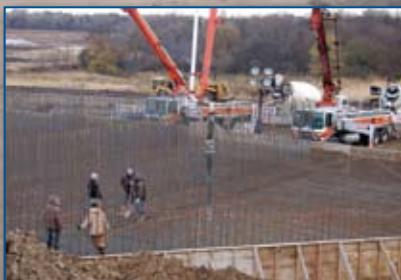
This forest of rebar waiting for concrete is the principal spillway inlet above the dam as it looked in early November 2009.
